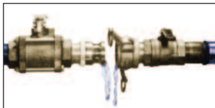
Ordinary Ball Valves Added = Spillage
